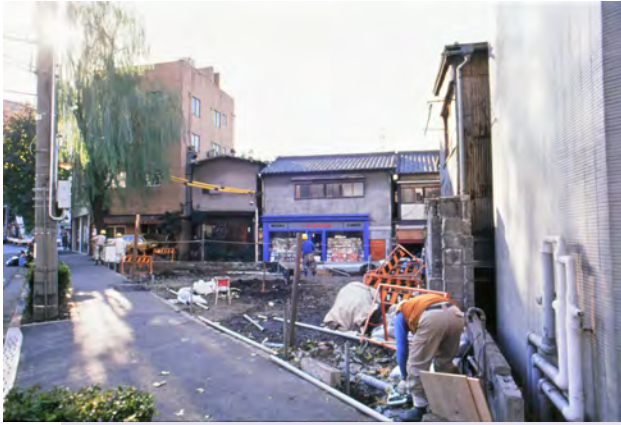
The site immediately after the demolition of the former Galerie Watari and On Sundays building. Preparing the fence around the site, end of November 1988.
