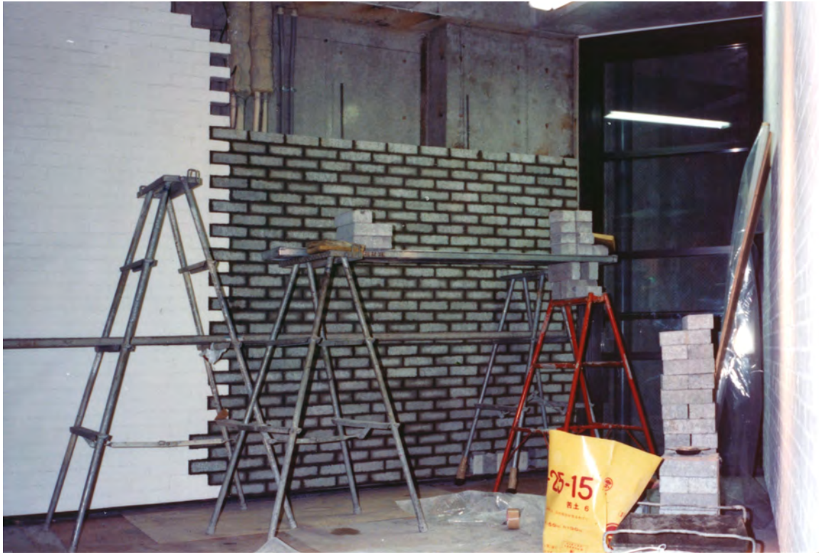
The exhibition space on the 2nd floor of WATARI-UM under construction. Custom-made concrete blocks being piled up to form an internal wall, spring 1990.
